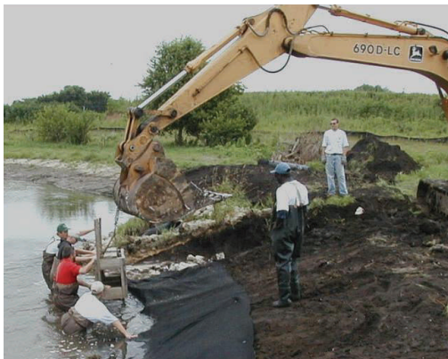
Lunkers, a type of bank stabilization and fish habitat improvement practice will also help retain property values for the sub-development adjacent to the stream.
