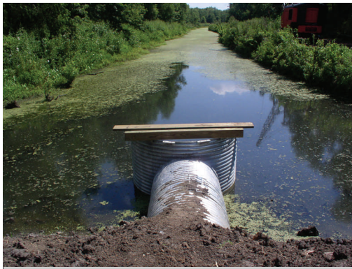
This structure is used to control water levels in a wetland that was added for enhance wildlife benefits for this landowner's CREP enrollment.
