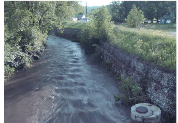
Peoria County: Gabion baskets filled with rock stabilize this open storm drain and prevent further erosion which would damage the adjacent street.
