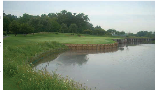
Bank Stabilization at Orchard Valley Golf Course. SWCD employees were responsible for performing construction reviews on the completed practices.
