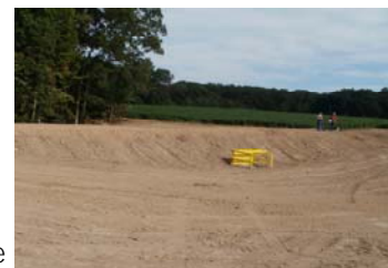
A trash guard is added and the new structure is ready for seeding
